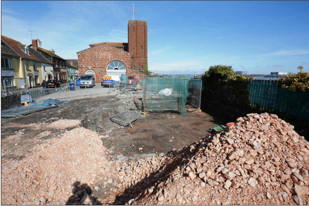
Plate 1: Site access behind Heras fencing to right of image. Engine house in background
