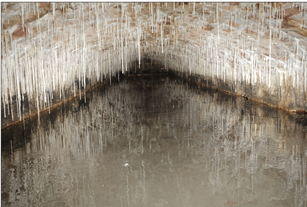
Plate 6: East chamber interior taken from north aperture. Tops of dividing wall arches visible to right above water level
