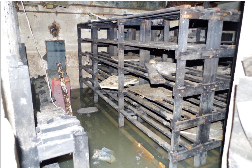
Plate 3: Interior detail of bunker showing extant structures and water ingress
