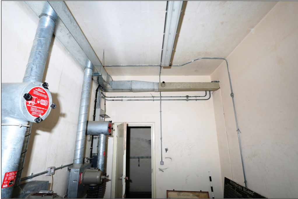
Plate 19: Plant room G showing reducer from new to old ducting
