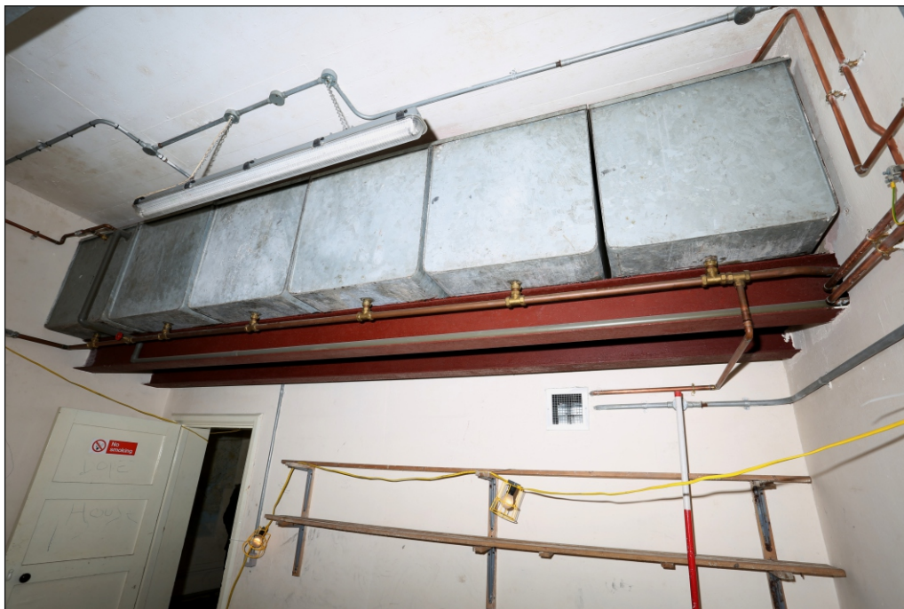
Plate 30: Kitchen M Water tanks
