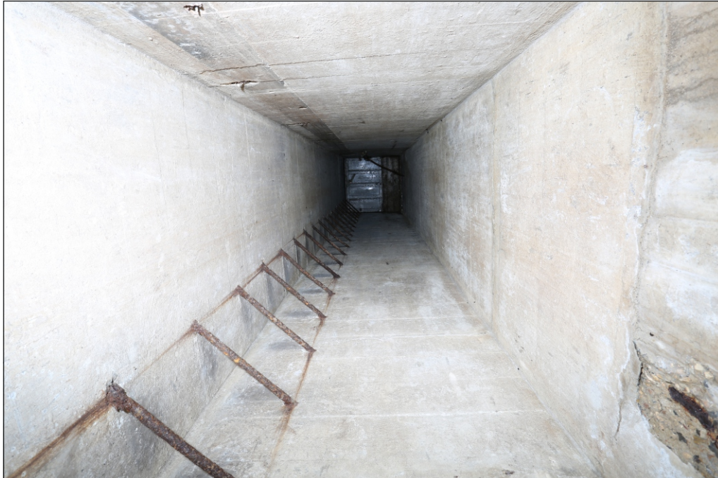
Plate 26: Escape shaft K looking up and showing angled ladder rungs set in concrete
