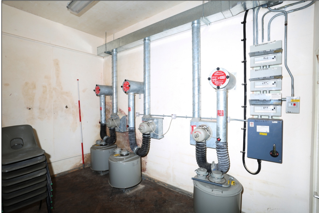
Plate 18: Air Ventilation plant room G showing modern circulation pumps
