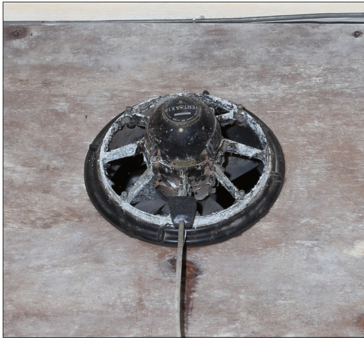
Plate 11: Vent-Axia extractor fan in generator room C
