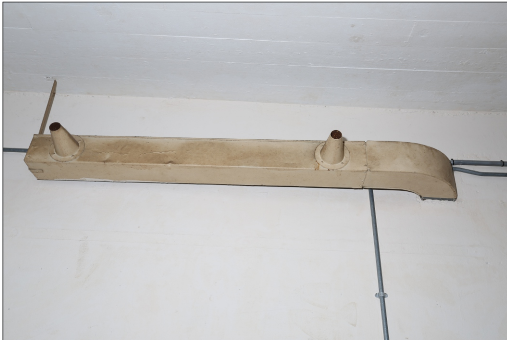
Plate 23: Control room I detail of cone air vents
