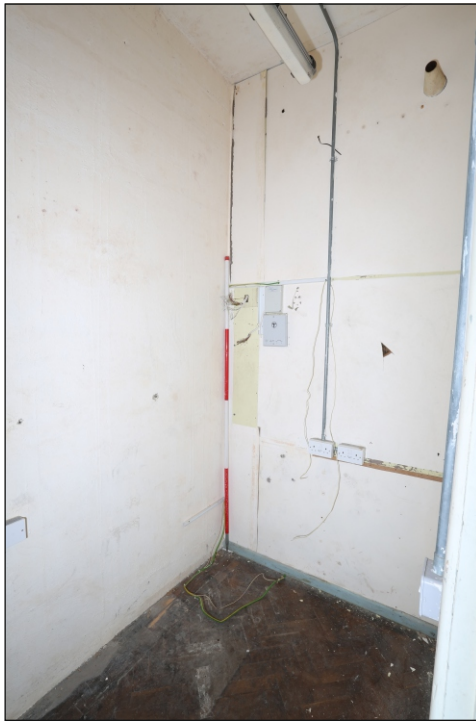
Plate 17: Telecom Room F
