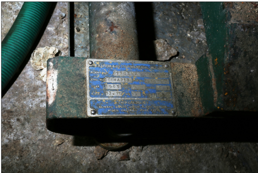
Plate 10: Generator diesel engine manufacturer's plate dated 1963
