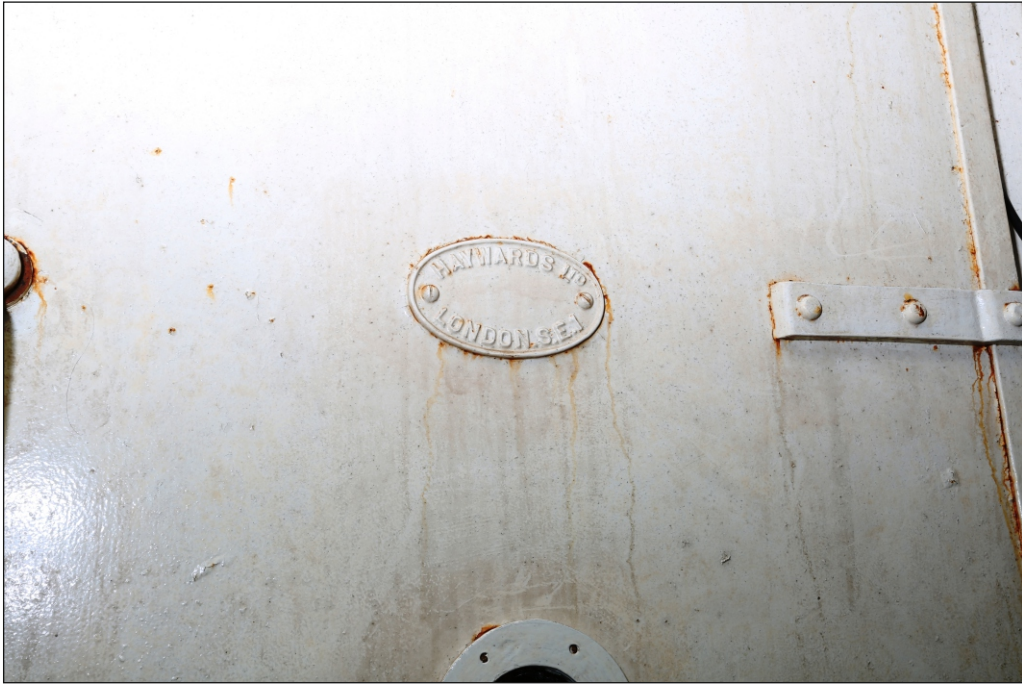
Plate 7: Detail of manufacturer's plate on sealable doors
