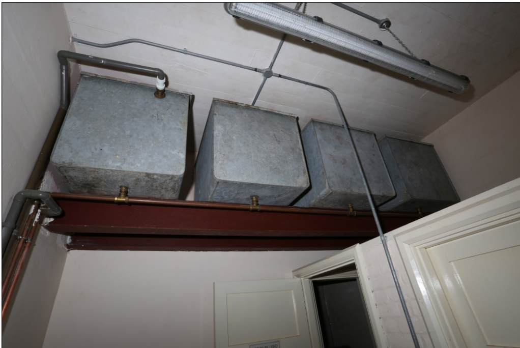
Plate 32: Water tanks in toilet N
