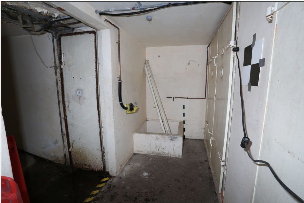
Plate 8: Decontamination shower base in lobby B
