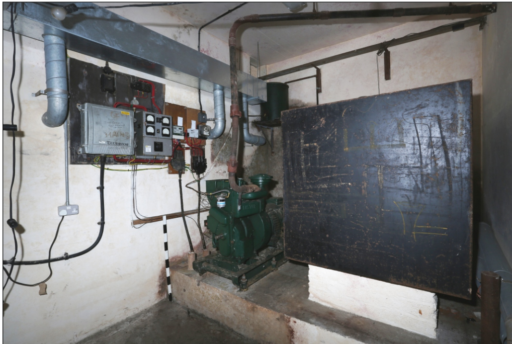
Plate 9: Generator room C showing fuel tank generator and switch board
