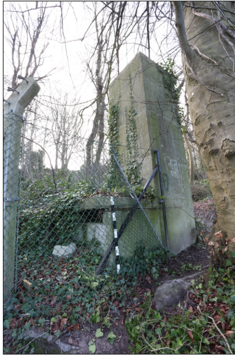
Plate 33: North-east concrete double vents showing low air intake and high level exhaust shaft
