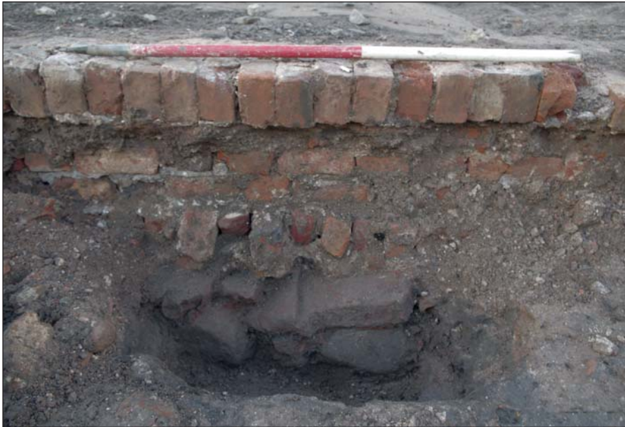
Plate 15: Brick wall 101 built on sandstone foundation 146 within construction cut 130. View from east
