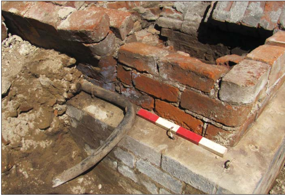
Plate 21: Bull nosed bricks ends on wall 1736 and vault 1735 and modern wall 1753 from the south-east
