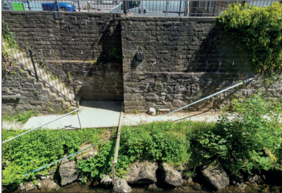
Figure 5: Access steps and iron railings in northern section of the river wall, view from the south-west
