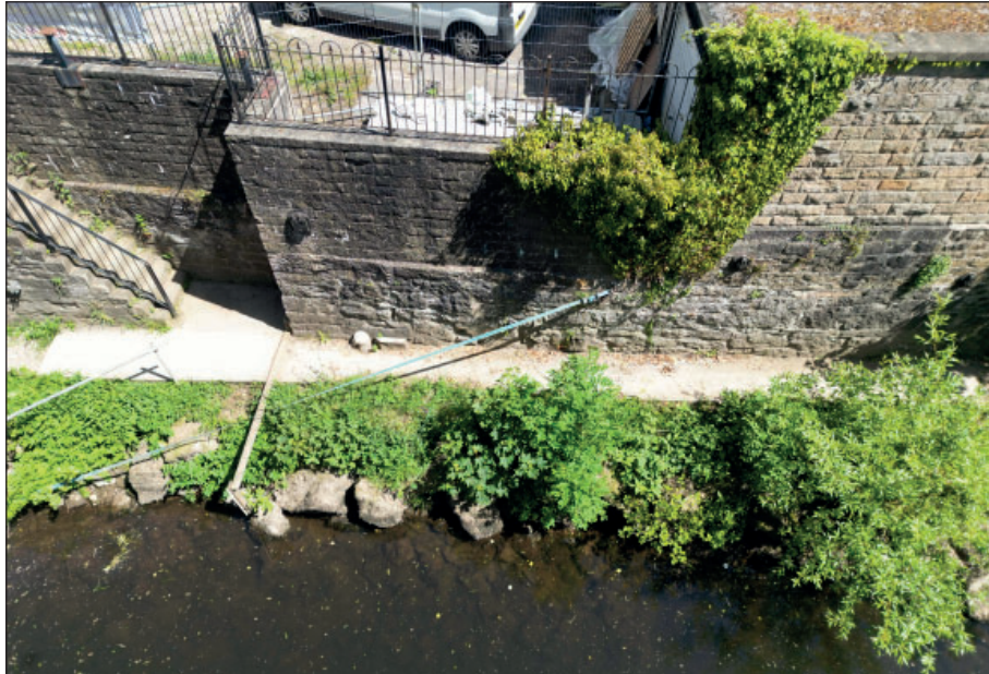
Figure 12: Access steps and ivy at the northern section of the river wall
