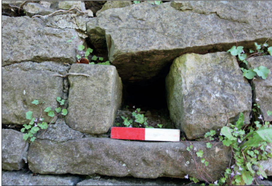
Figure 7: Drainage hole in the southern section of the river wall, 0.2 m scale
