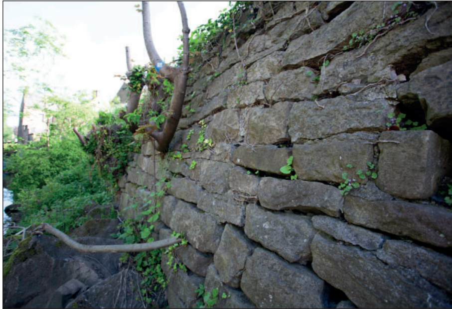
Figure 9: Medium-sized tree in the southern section of the river wall
