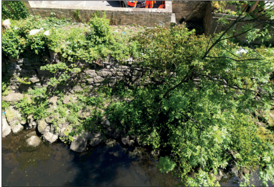
Figure 11: One medium-sized tree and vegetation growth at the middle section of the river wall
