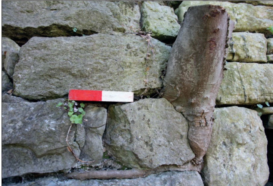
Figure 8: Small tree in the open joint of the southern section of the river wall, 0.2 m scale
