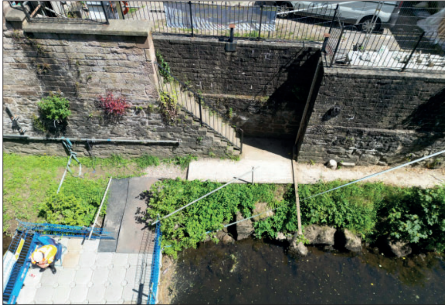
Figure 13: Access steps and vegetation growth at the northern section of the river wall
