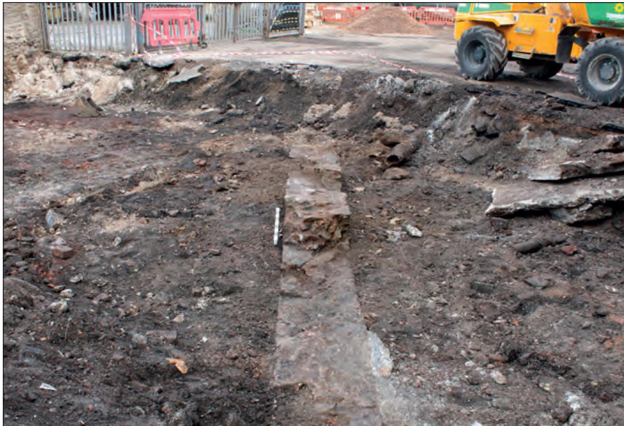
Figure 40: Stone wall foundation (4048, group 1083) on north side of retort house, looking east. Scale: 1 m (photograph by C. Mason).
