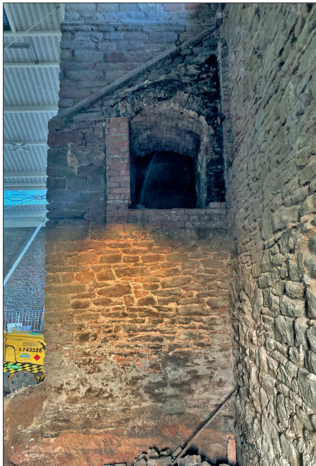
Figure 74: High level flue opening into the coal store chimney, looking north-west (photograph by C. Mason).
