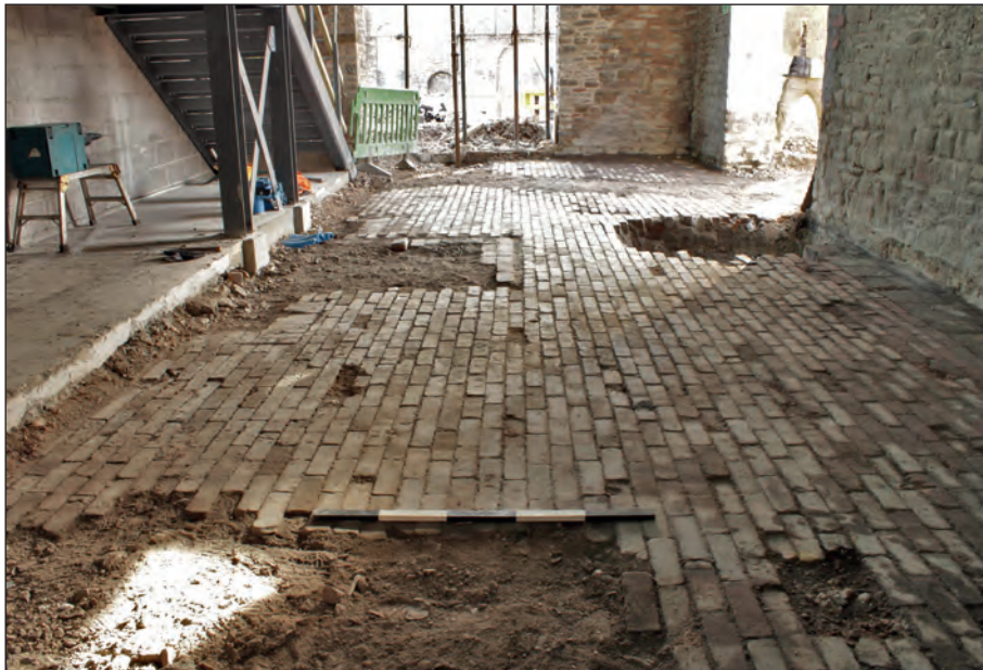
Figure 95: Brickwork at south-west end of cooker incinerator (group 3060) and brick floor (group 3055) in the north-west range of the retort house, looking south-east. Scale: 1 m (photograph by C. Sabato).
