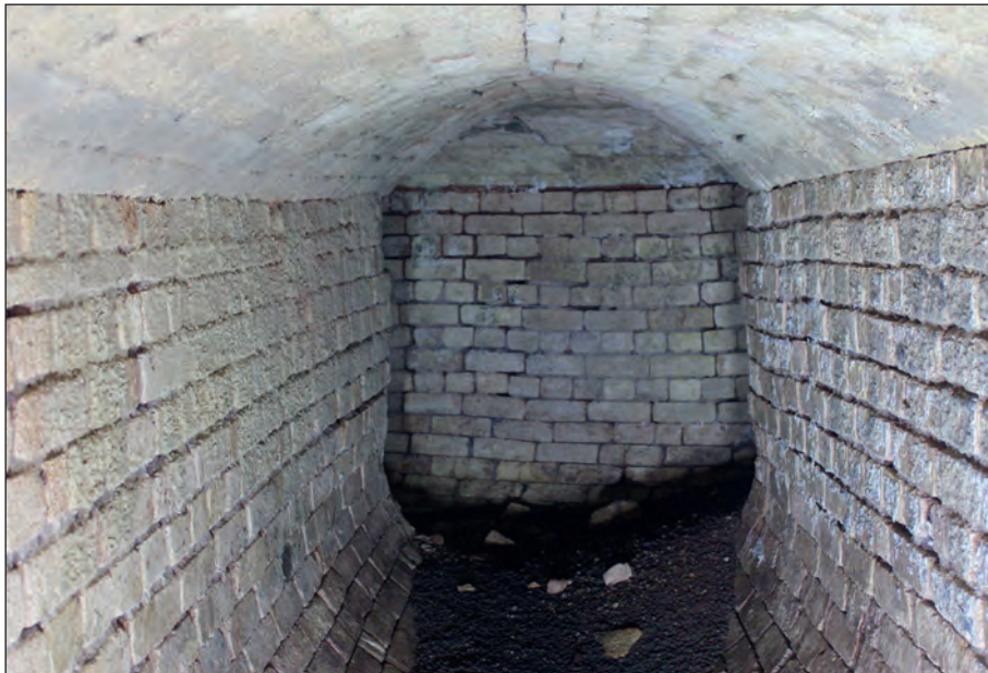
Figure 71: Internal view of flue (group 1084) in coal store, looking north-east (photograph by C. Mason).
