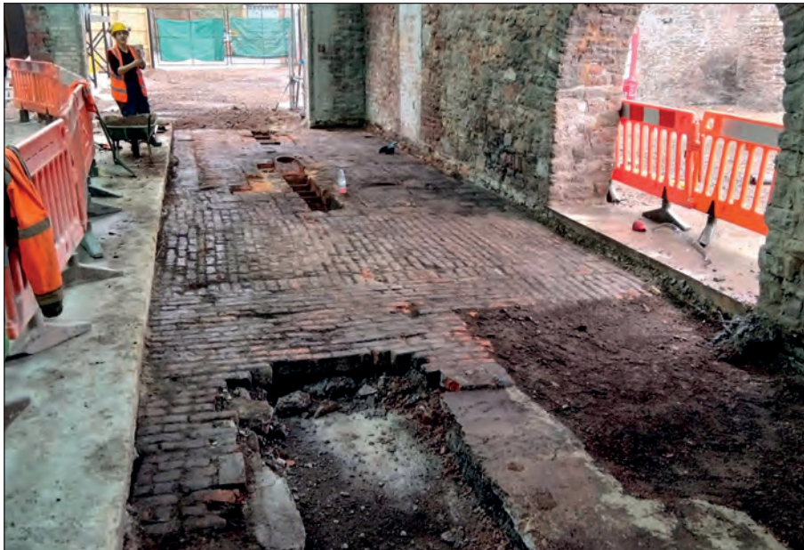
Figure 50: Retort bench (group 3058) and brick floor (3041–3) at the north-east end of the north-east range of the retort house. Looking east (photograph by A. Pannell).
