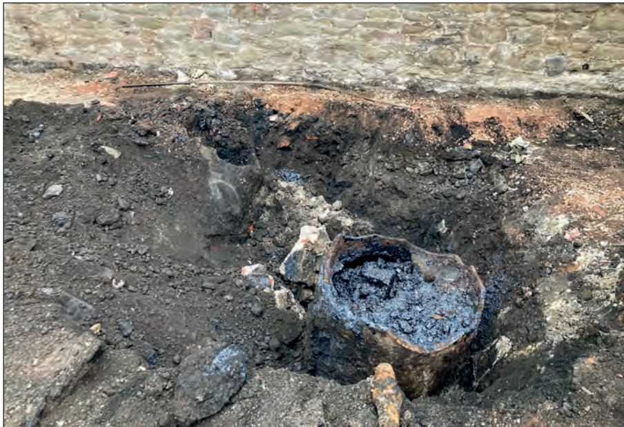
Figure 101: Gas pipe 4034 filled with coal tar oil. Looking north-east (photograph by C. Mason).
