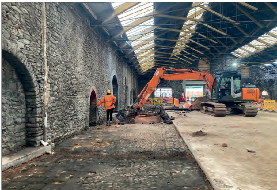
Figure 75: Fireclay slab and sandstone sett floor (group 1082) on the south-east side of the coal store, looking south-west (photograph by C. Mason).
