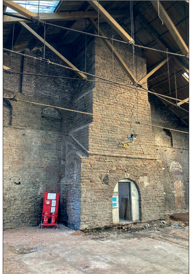
Figure 47: Chimney at north-east end of coal store, looking east (photograph by C. Mason).
