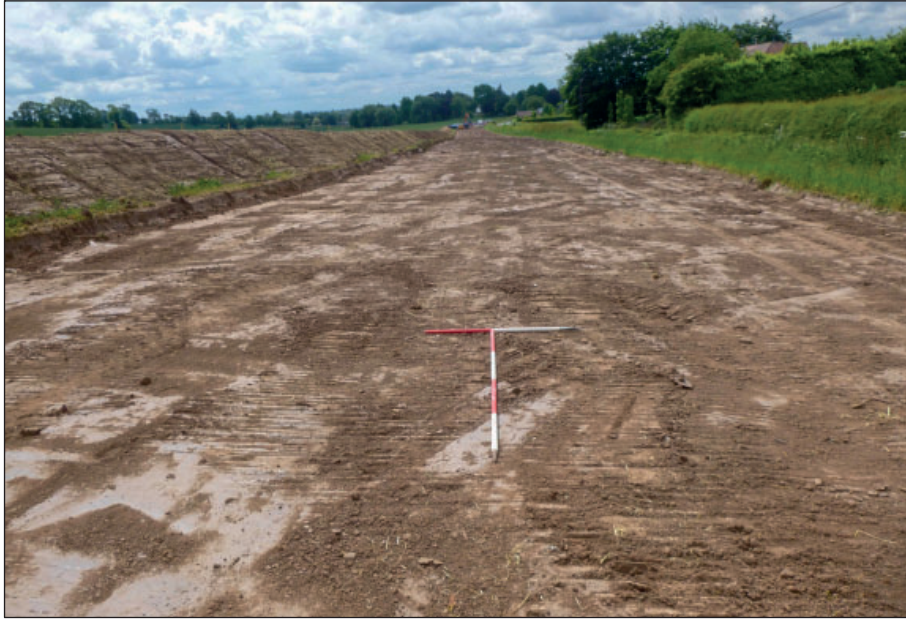
Figure 2: Topsoil strip, east of Chapel Lane, south end of stripped area, view from north, 1 m and 2 m scales
