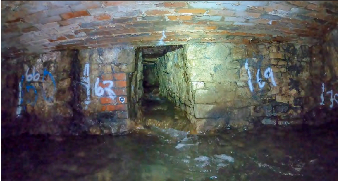
Photograph 24: The lateral channel that runs south under 4 Leg Square and presumably further under the Square (67m chainage)
