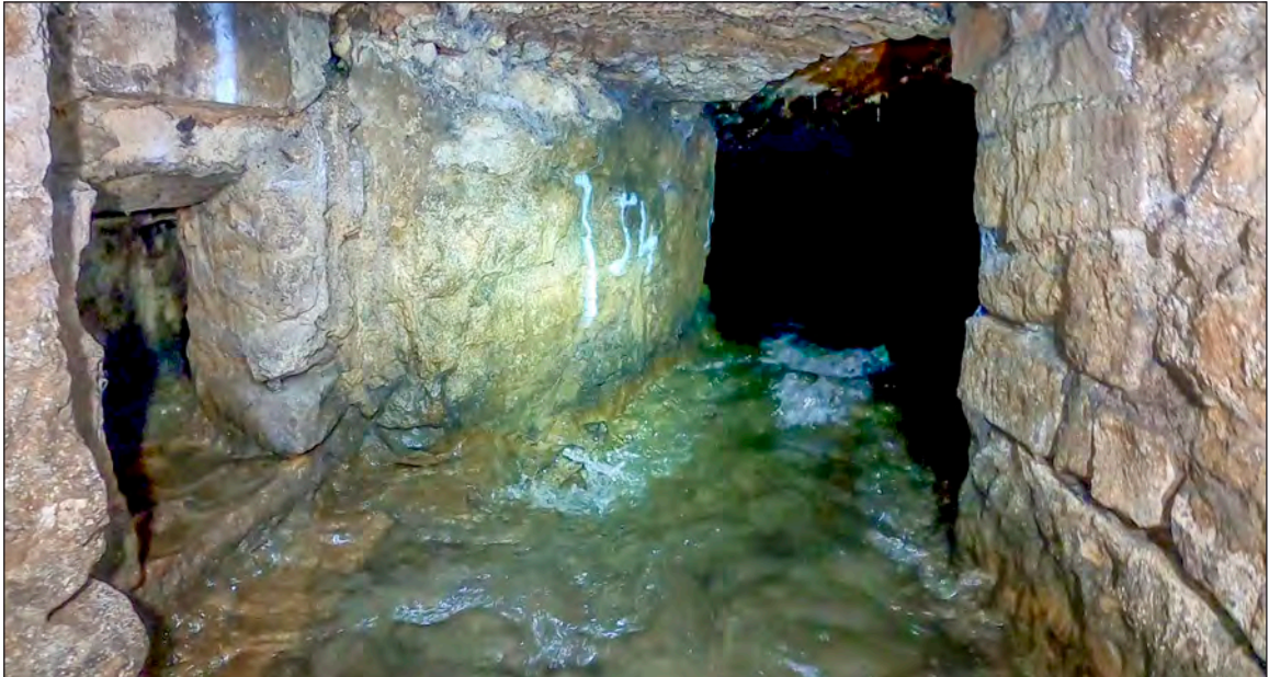
Photograph 20: The west end of bifurcation left with a lateral connecting channel or leat on the left (52m chainage)
