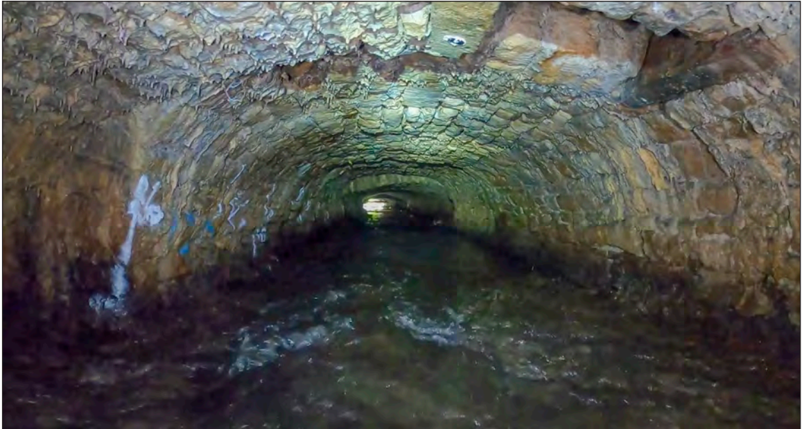
Photograph 26: The narrow part of culvert towards its western end (86-93m chainage). Note the multiple variations in the size and shape of the arch. A possible manhole cover is visible top right.
