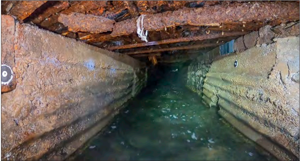
Photograph 1: Inaccessible concrete lined and re-roofed part of the southern channel from the inlet
