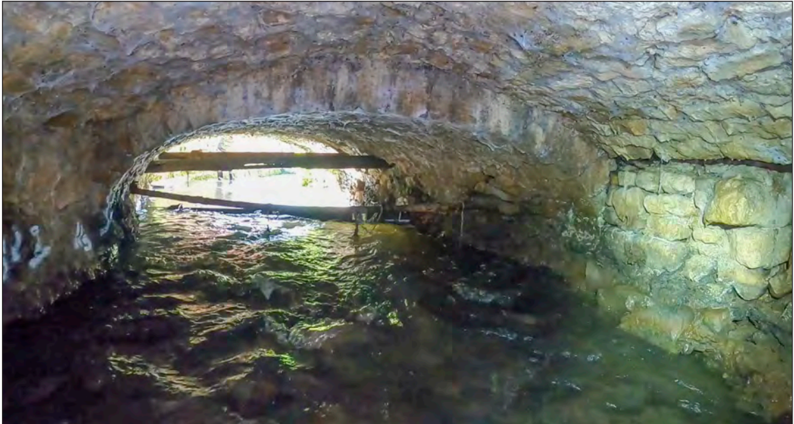
Photograph 30: The western end of the culvert partially blocked by pipes and cables (113m chainage)
