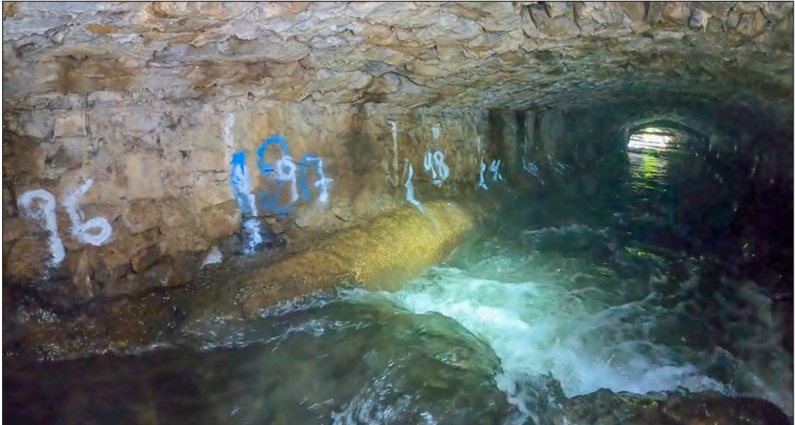
Photograph 28: Another drop structure (97m chainage) and the concrete plinth built along the south wall of this part of the culvert
