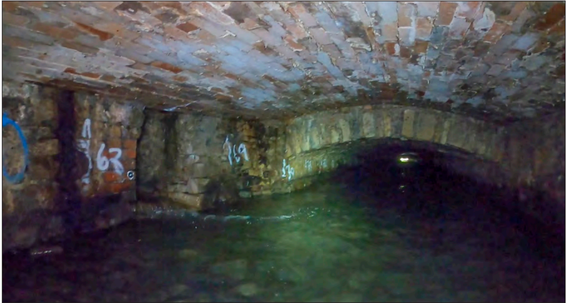
Photograph 23: Photograph showing the change from a brick soffit to a lower stone arch, plus a lateral channel or leat on the left (c.67m chainage)
