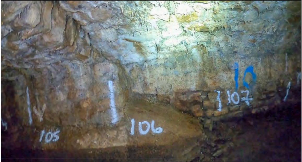
Photograph 29: The western end of the concrete plinth as the culvert widens again (106m chainage)
