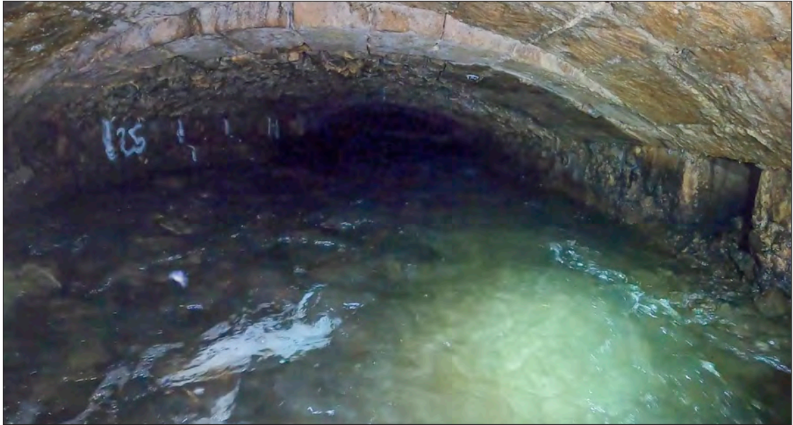
Photograph 13: A change in soffit material from limestone ashlar blocks to stone rubble and drop in the arch as the culvert crosses under the street (24.5m chainage)
