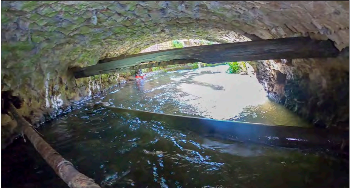
Photograph 31: The western end of the culvert partially blocked by pipes and cables (113-118m chainage)
