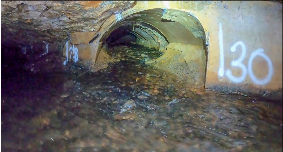
Photograph 15: The stone arch culvert which may be a leat associated with the Old Flour Mill, Leg Square (town mill, HER no. 11078; 29m chainage)
