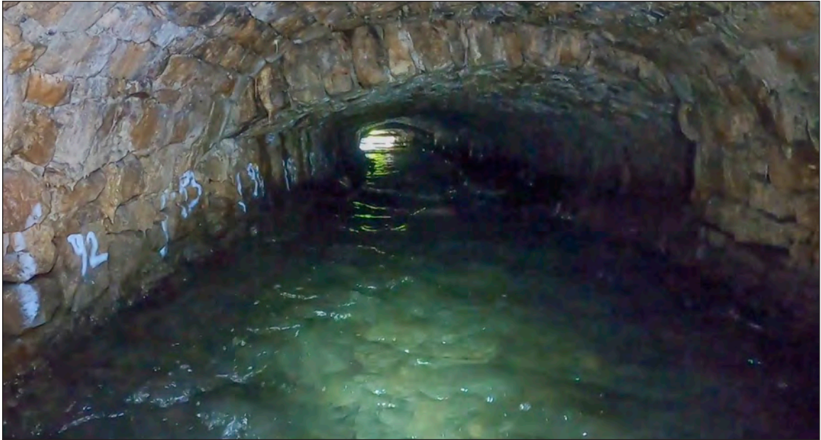
Photograph 27: Another change to the size and shape of the culvert (from 93m chainage)
