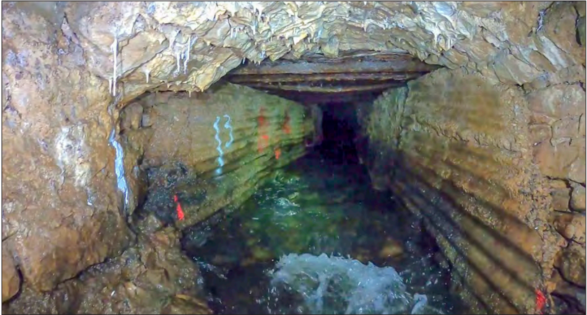
Photograph 5: Another concrete-lined and metal-roofed section towards the western end of the southern channel from the inlet
