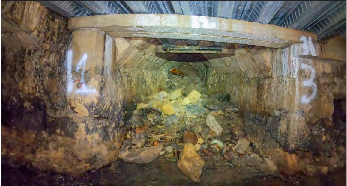
Photograph 11: The drain from the mill leat on the south side of the junction chamber
