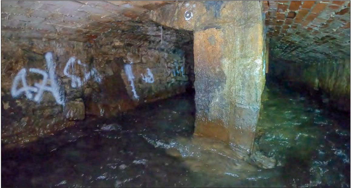
Photograph 17: The stone wall which divides the culvert into bifurcation left and bifurcation right (c. 47m chainage)
