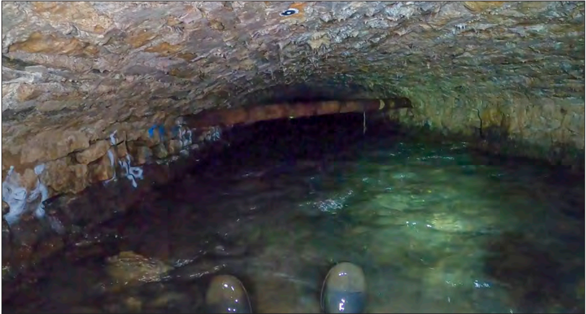
Photograph 25: A pipe crossing through the culvert (c. 78m chainage)
