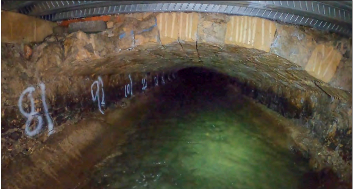
Photograph 12: View looking west along the culvert from the junction chamber (8m chainage)
