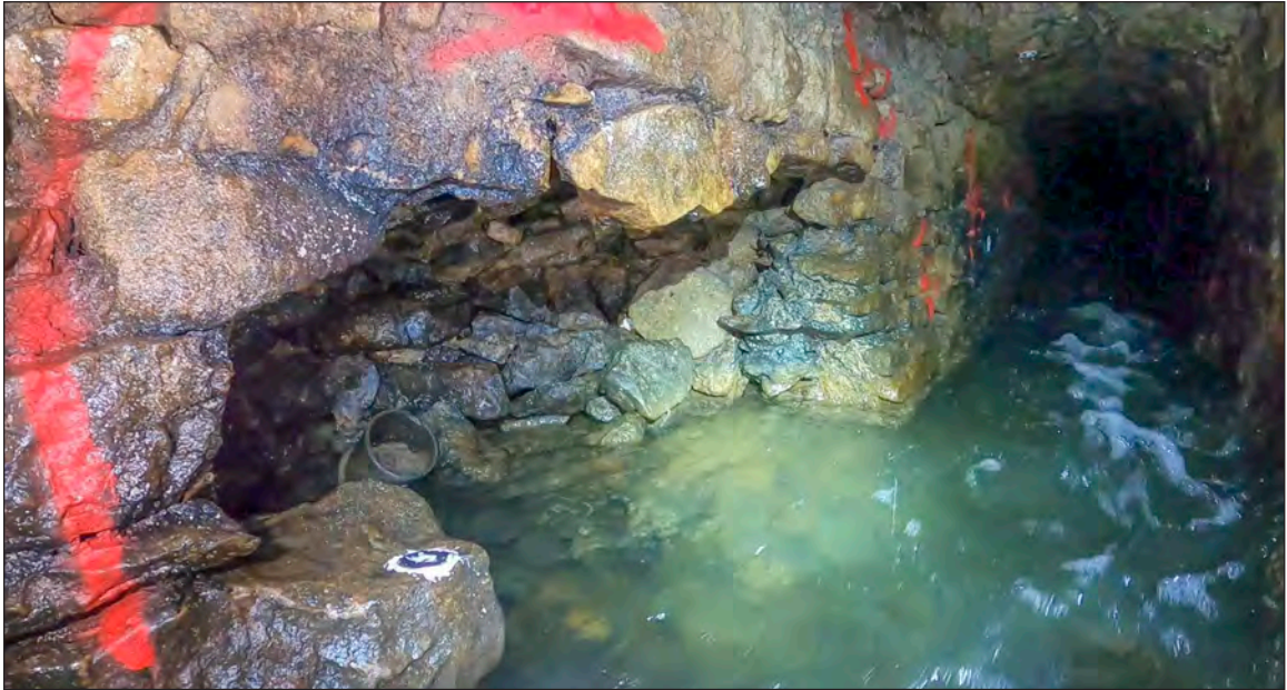
Photograph 3: Example of the scouring which has undercut the southern channel at the east end of the recorded culvert
