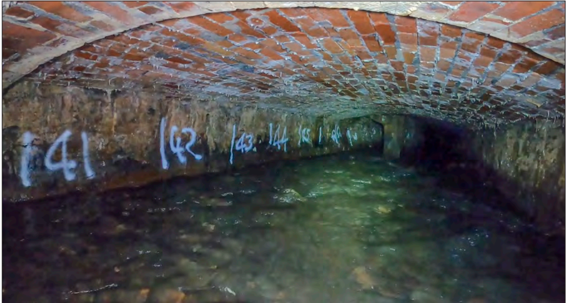
Photograph 16: A view looking west towards the bifurcation showing that the soffit has changed to brick (40.5m chainage)
