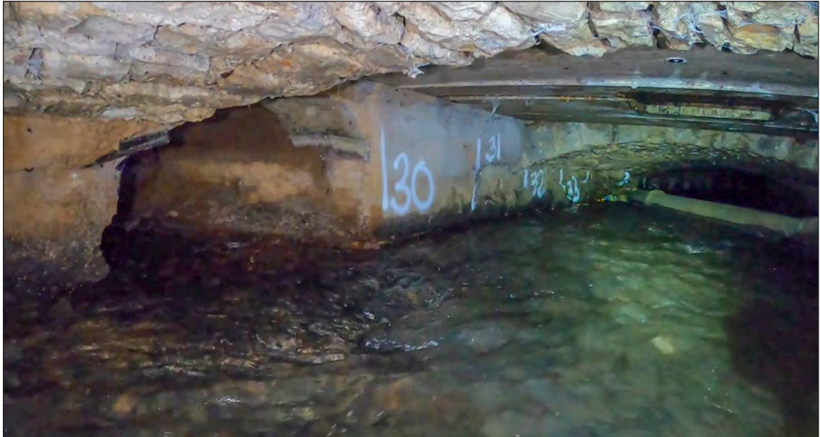
Photograph 14: A concrete section of the culvert under the street carriageway, with a smaller stone culvert joining from the south (left) (29.5m chainage)
