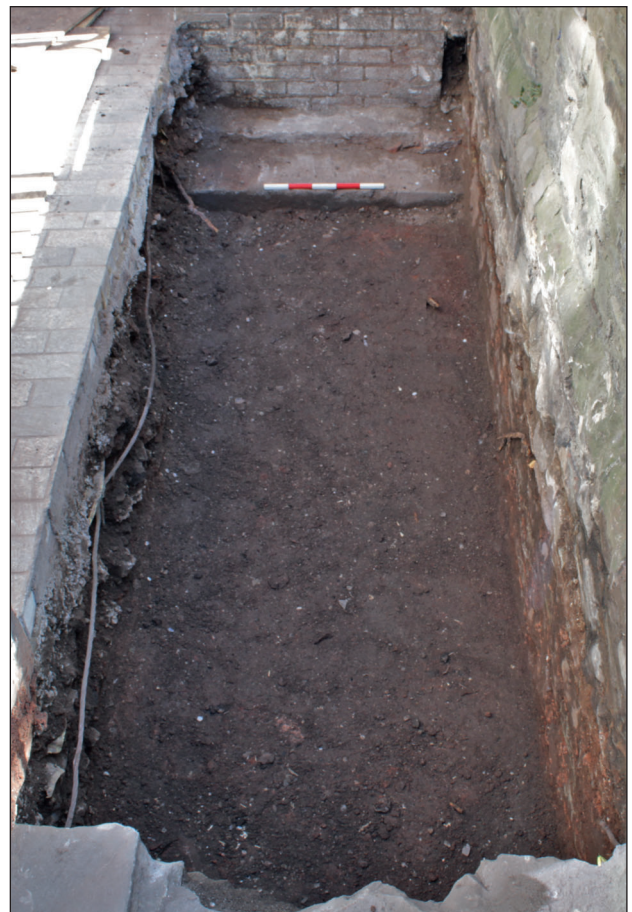
Figure 6: Trench for new steps in John Street, looking north-east, scale: 0.5 m (photograph by C. Hambleton)
