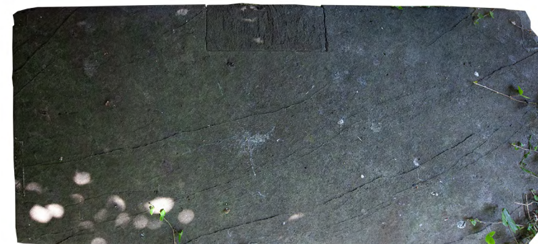
cut out decayed stone and allow for indentation of new corner of tomb lid, in new oolitic limestone, nominally 140 x 135 x 40
