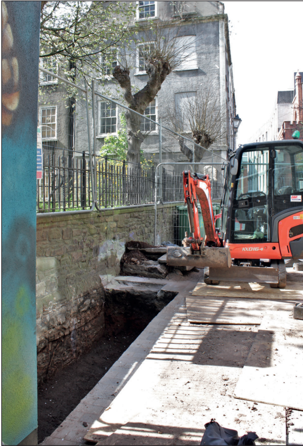
Figure 5: Trench for new steps in John Street, looking south (photograph by C. Hambleton)
