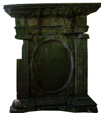
resecure loose element of pilaster; see details below
