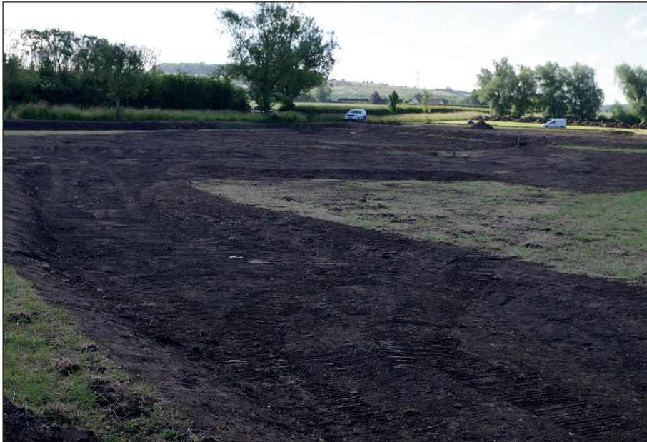
Figure 4: General view of northern extent of ground reduction for the basin, view from the north-west
