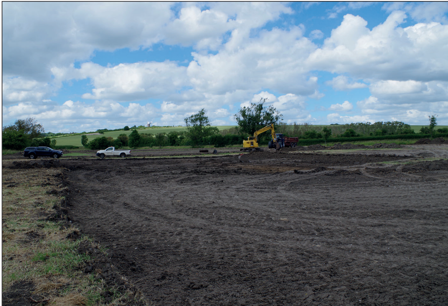
Figure 5: Ground reduction for the southern extent of the basin, view from the north-west
