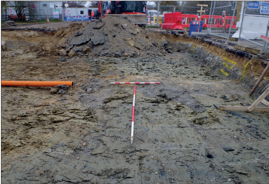
Figure 4: Trench 5 from the south-west, scales: 1m and 2 m (photographed by S. Froud)
