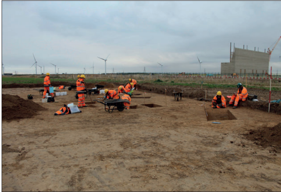
Figure 206: Area 61, view from the south-west, Bicker Fen substation under construction in background
