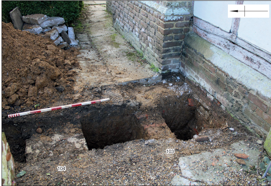
Figure 7: House foundations (right) and walls 103 (centre) and 104 (left), 1 m scale, looking east
