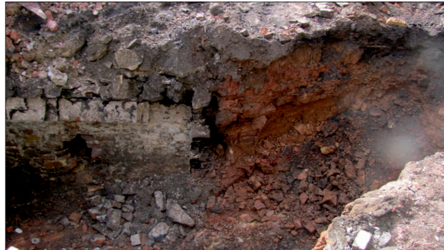
Plate 14: Watching brief trench 19 from east with wall 1903 removed to show construction cut 1914 containing wall 1901
