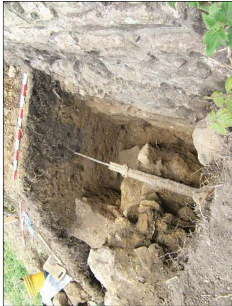
Plate 1: Cut for electric cable and disturbance of wall 106 by robber cuts 103 and 111, view from west
