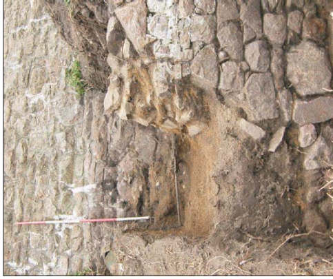
Plate 16: Disturbance of wall 106 and base wall of the Grand Battery 116, view from north-east
