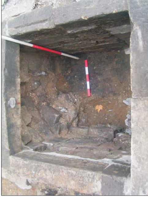
Plate 5: Remains of Tudor stairwell 137 in the north-facing elevation of Victorian cellar entrance chamber 110
