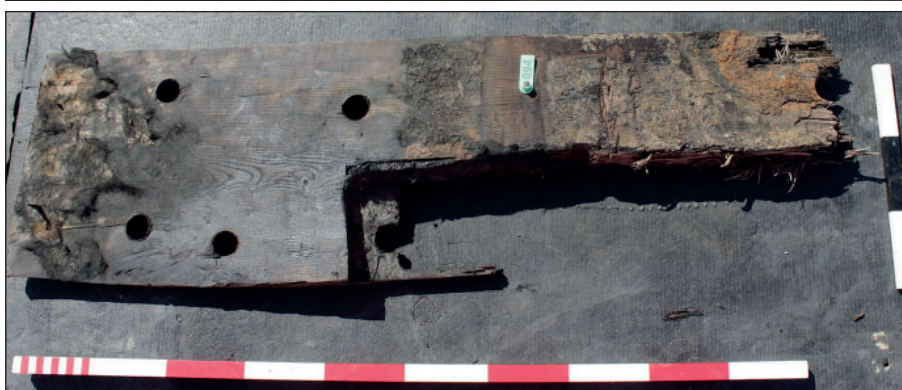
Figure 44: A large wedge sat on top of this repair. The fact that the waterproofing material was removed from the patch suggest that this repair was done before the insertion of the filler frames
