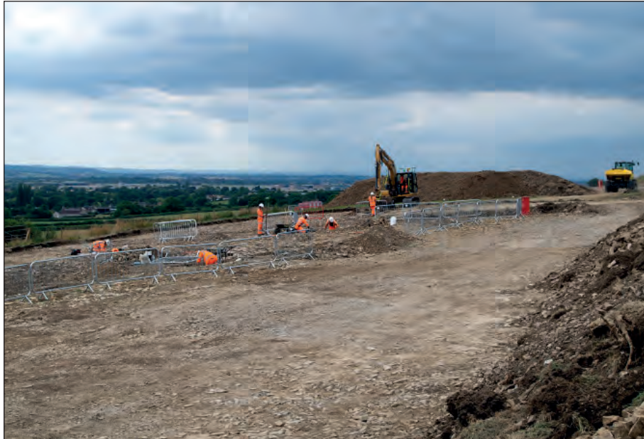
Figure 5: General view of SMR05 excavations, from the north-east (photograph by A. Misiak)
