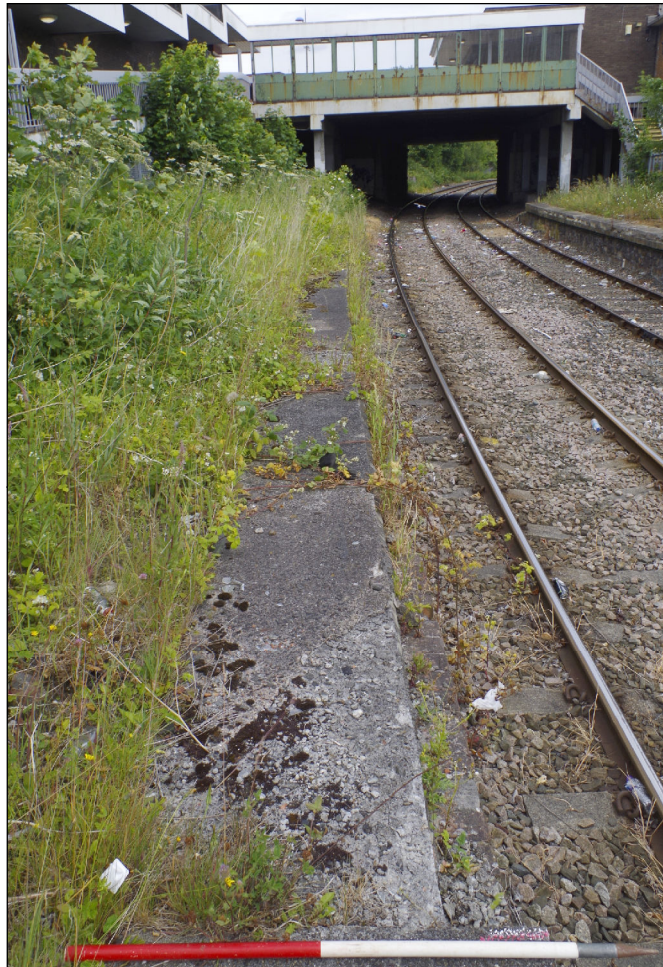
Photograph 4) View of the concrete slab on the northern section of the West Platform, facing north
