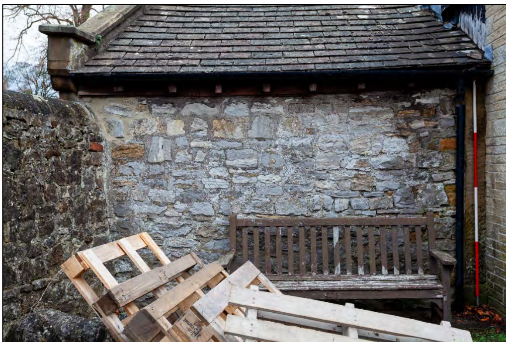
Plate 8: Possible infilled bay to the western end of the Cart House, facing north
