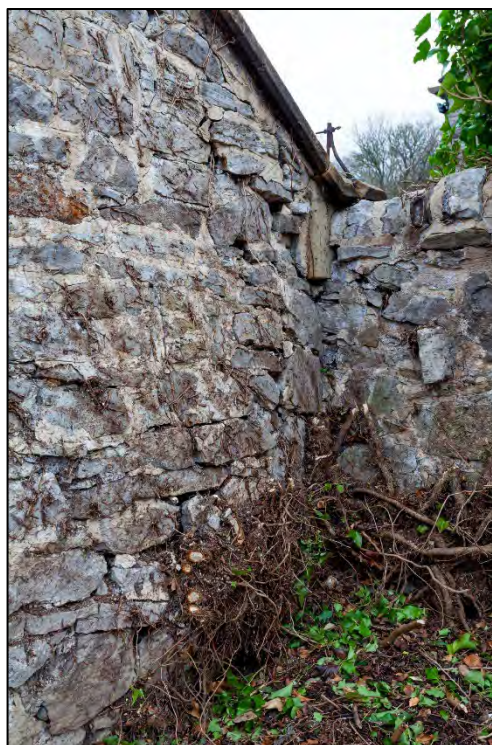
Plate 16: Displaced stonework to the east side of the Cart House, facing northwest
