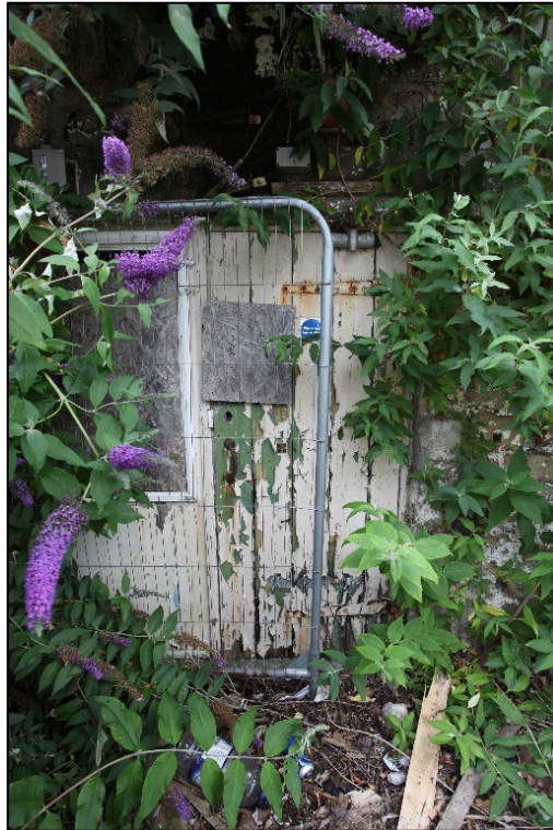
Plate 15. Original double-width doorway with later door and window to the building's eastern elevation
