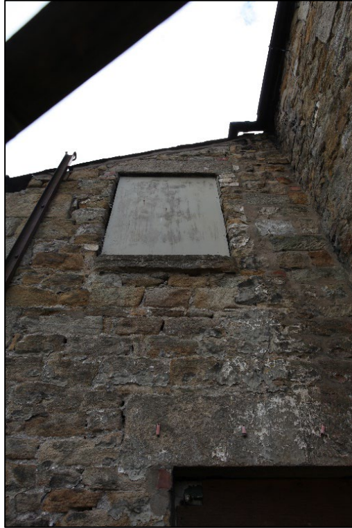
Plate 11. Original window opening to first floor level, at the east end of the north elevation
