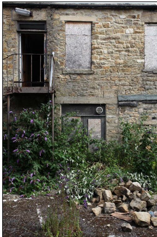
Plate 4. Doorway to ground floor, west elevation, with altered window opening and inserted fire escape door above
