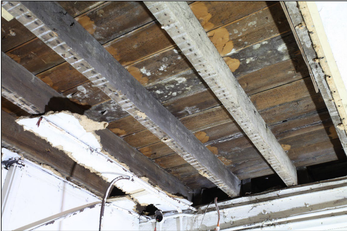
Plate 21. Detail of first-floor floor construction with evidence of former lath and plaster, facing north-east within the lobby
