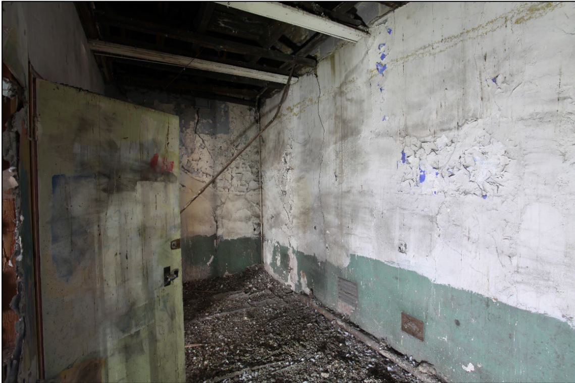
Plate 39. Overview of room 6, seen through a hole in the stud wall partition to room 5, facing south-east
