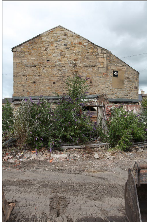
Plate 17. South elevation of the building – note the intersection of the infill extension with the main block
