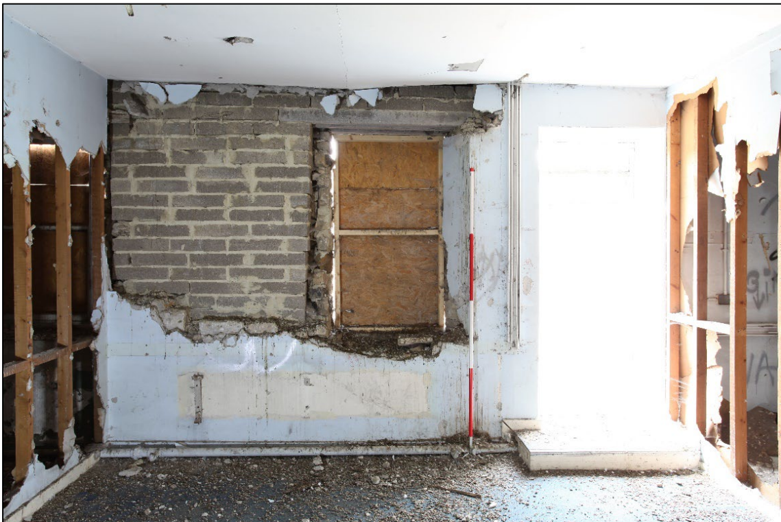
Plate 38. Detail of extensive recent repair work to the west wall of the building, within room 5, facing west
