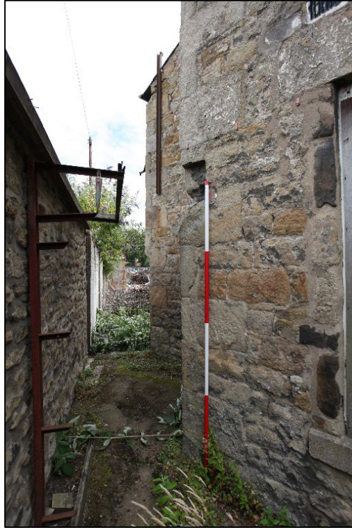
Plate 9. East corner of the north end of the main block – note the hacked-out void/mortice for a former extension to the building
