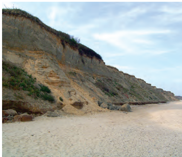
Plate 4.1 Eroding cliff at Pakefield, Suffolk
