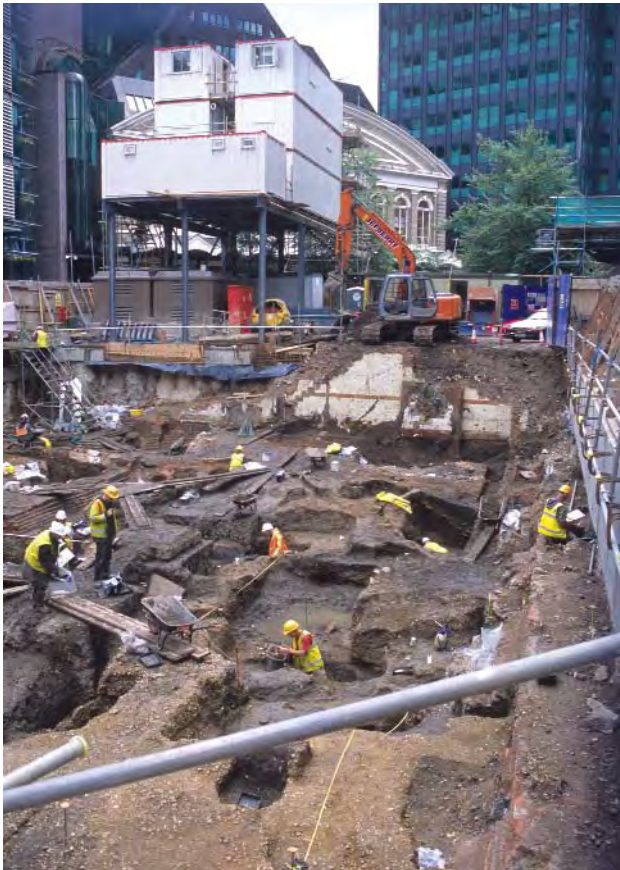
Figure 3 Excavation in progress in the rear of the plot, with Fenchurch Street Station in the background. The lighter coloured gravel layers of the Roman roads are visible in the foreground
