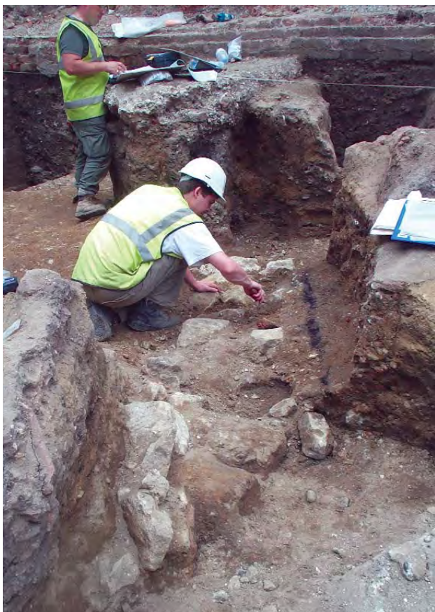
Figure 26 Period 6 Building 14: construction detail of the north-west wall showing roughly hewn ragstone blocks bonded with pale grey mortar above the remains of wooden piles
