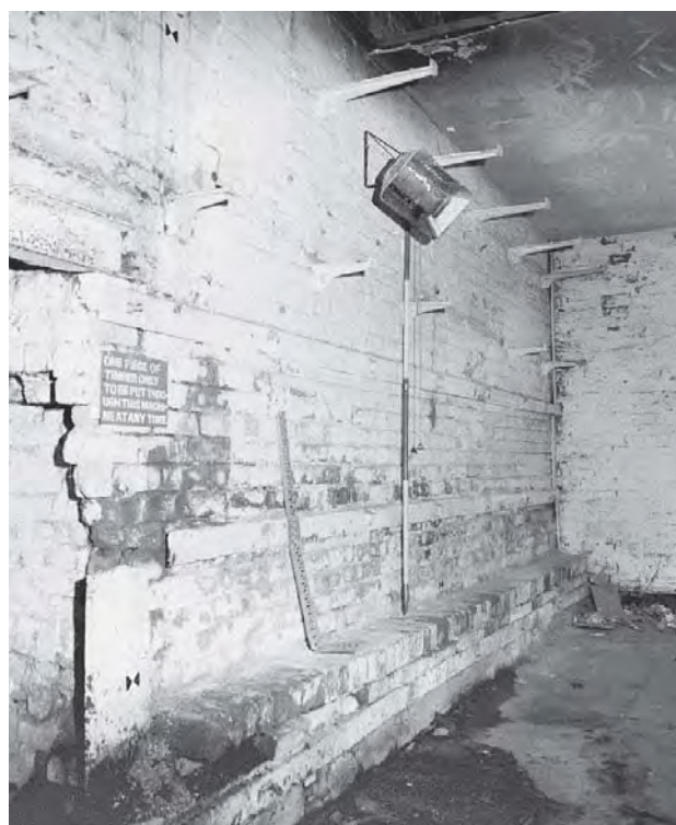
Figure 41 Titanic Works, building F1, detail of south-east crucible stack, showing ledge and shelf brackets
