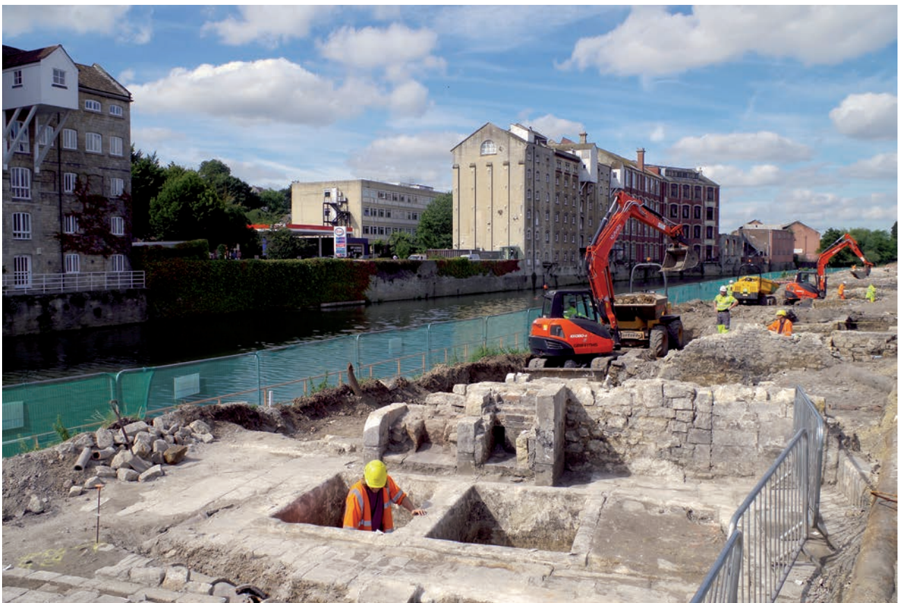
Plate 1.6 Excavation of stone-lined liming pits within an 18th-century fellmongers and parchment works at 3 New Quay (view from the north-east), with Camden Malthouse, Camden Mill and the Albion Stay Factory in the background
