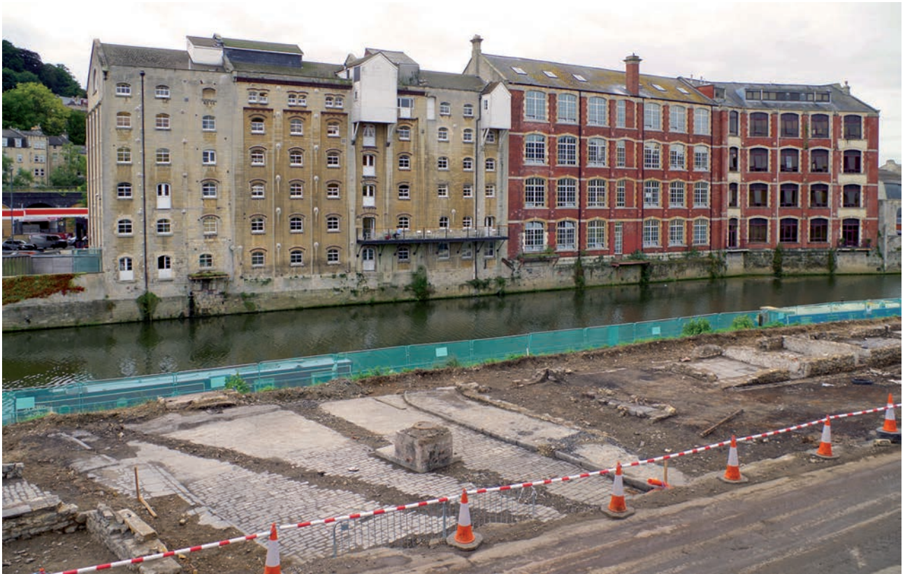
Plate 1.5 Avon Street, viewed from the north-east, with Camden Mill and the Albion Stay Factory in the background
