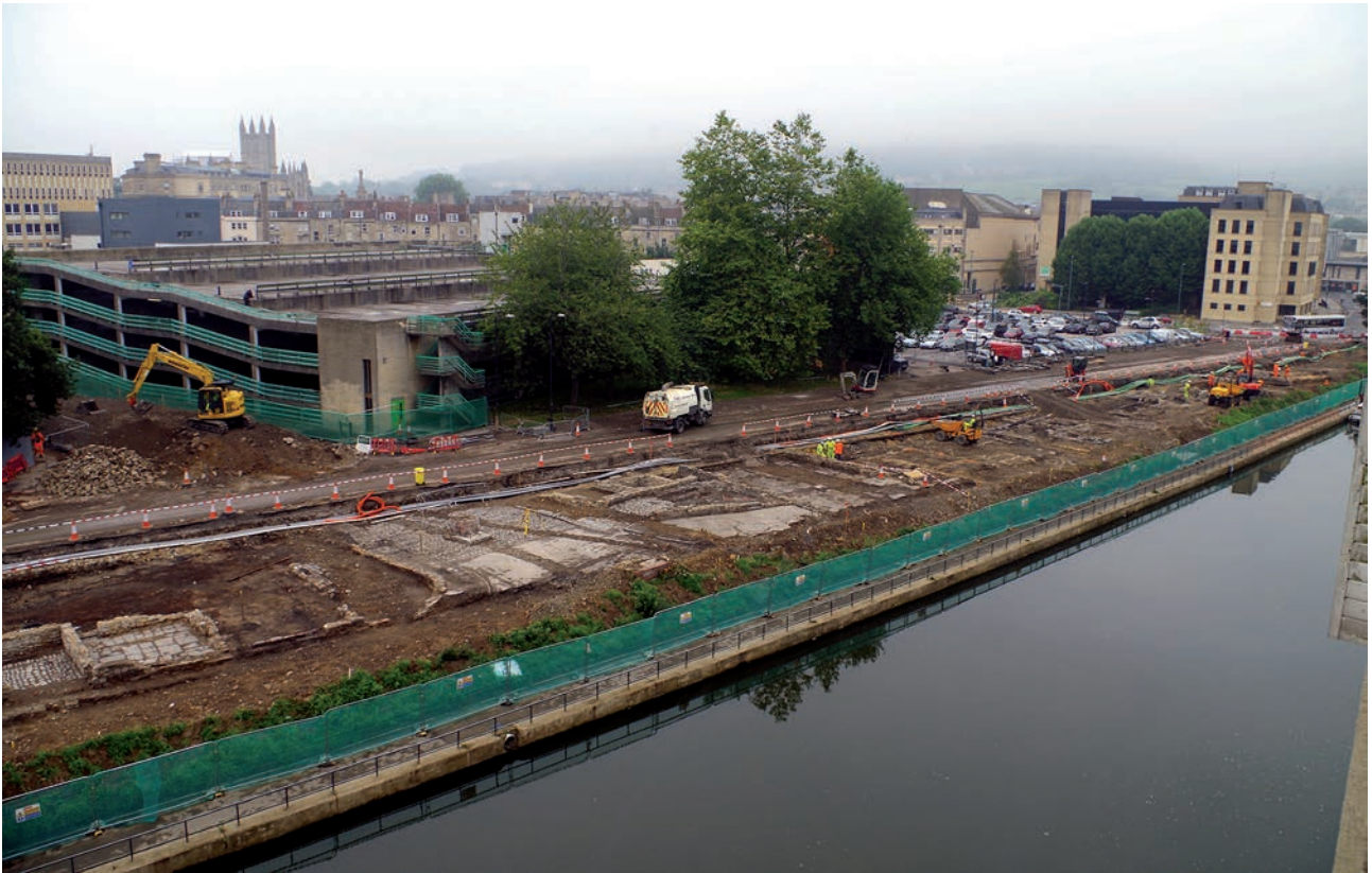
Plate 1.3 Excavation area from the west, showing the excavated remains of buildings along Avon Street and New Quay, with Avon Street multi-storey carpark in the background
