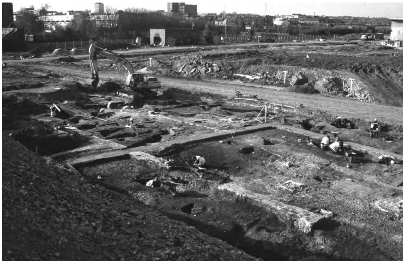
Figure 39 View of machine clearance in progress in the South Stand area, looking north-west
