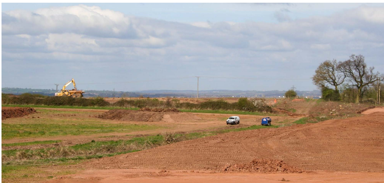
Plate 2.12 Topsoil stripping of the Mill Close site, as seen from Seven Geaves
