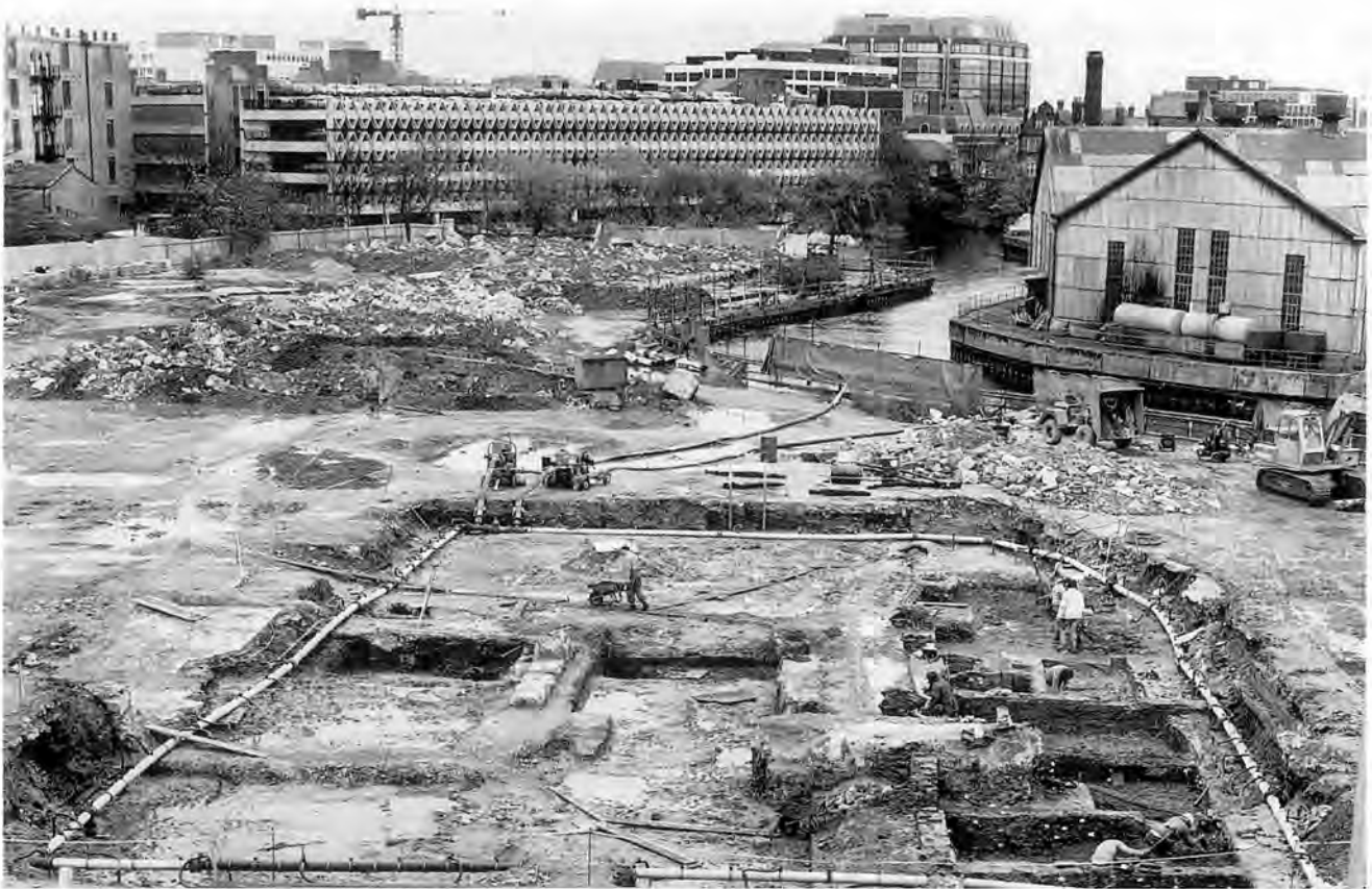
Plate 1 The well-point dewatering system in operation at Bridge Street East (site W158). Individual small wells secured to the end of riser pipes are inserted at approximately 1 m intervals into the relevant permeable stratum under high water pressure. The riser pipes are connected by a swing connection to a header pipe, in turn connected to a well-point vacuum pump. The effect is to produce a dry core around each well-point thus preventing groundwater from entering the excavation.
