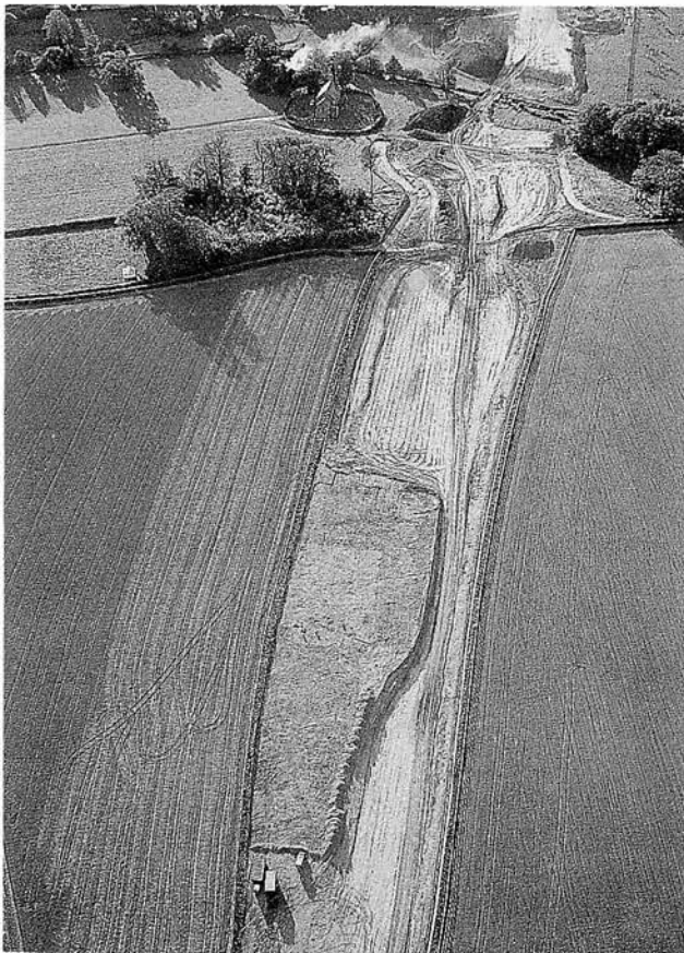
Plate 13 Languard Lane: the excavation, viewed from the east, surviving as an 'island' amongst the earth-moving. The River Tale, church of St Philip & St James's and woods of Fairmile are in the distance. Photograph (29 October 1997) by Bill Horner, Devon County Council. Copyright reserved
