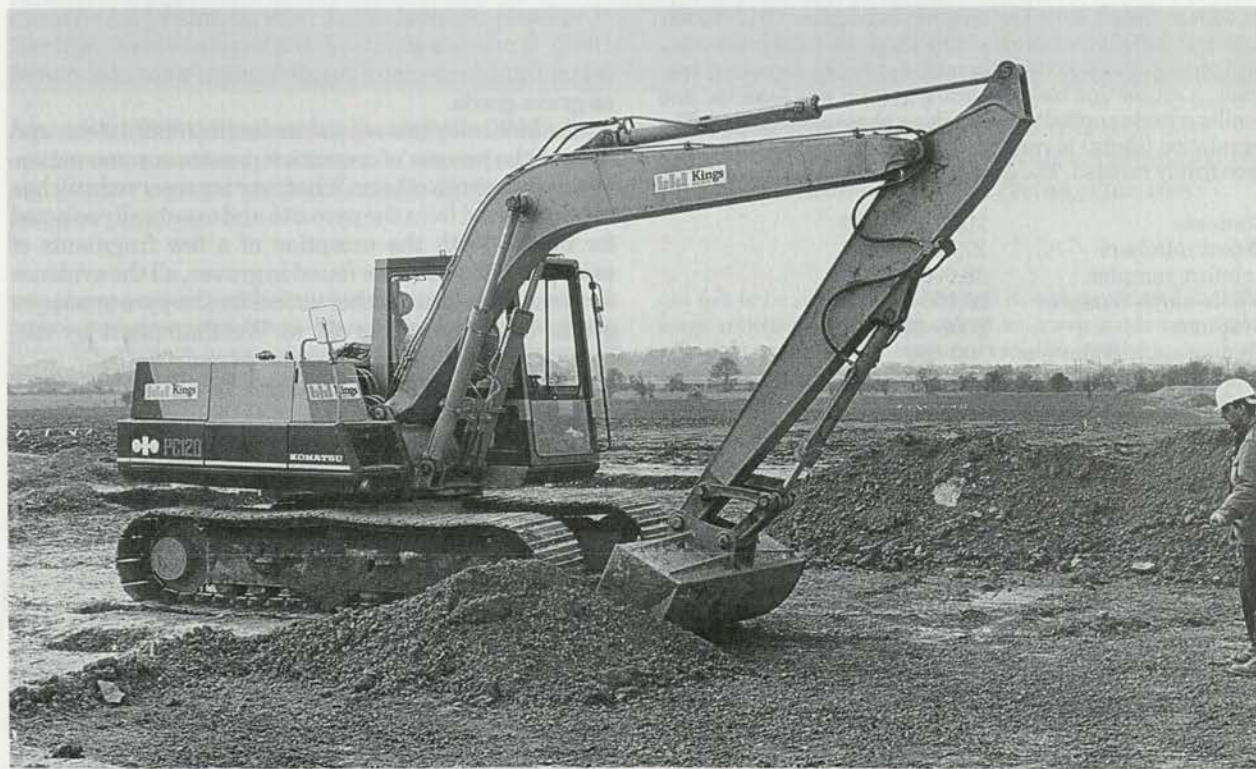
Plate 4 Supervising the final machine cleaning of the excavated Iron Age cemetery in order to remove any of the reworked loam sealing features cut into the natural gravel. Note the excavated graves beside the excavator. The view to the south-west includes the edge of Area 3 to the right
