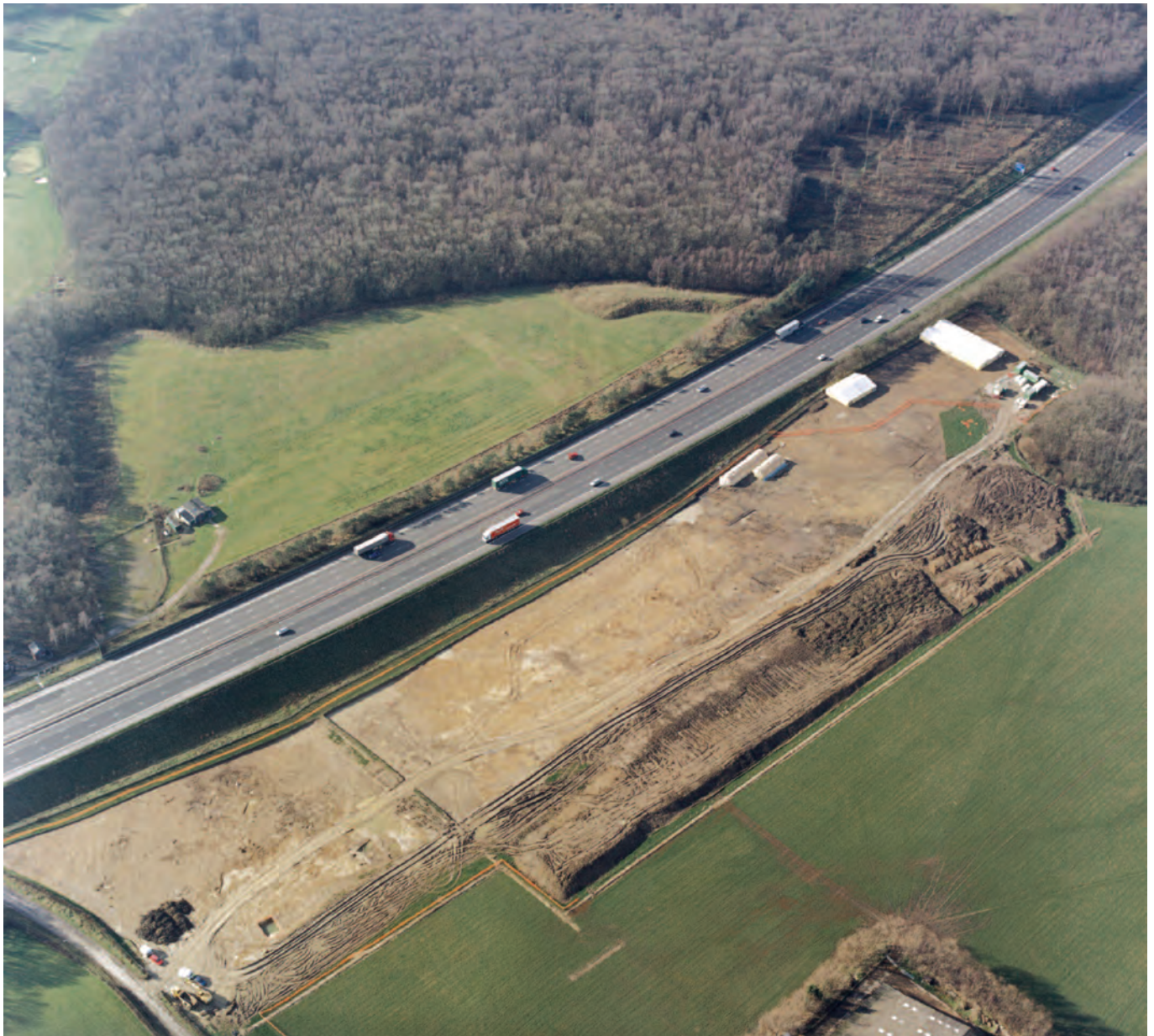
Figure 1.2 Thurnham Villa aerial view of excavations in progress. Roman buildings covered with marquees and polytunnels
