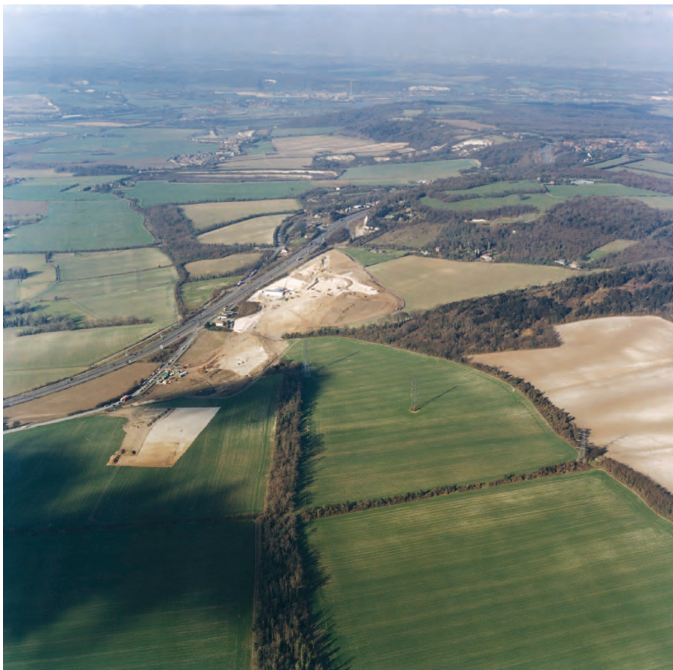
Figure I.1 High Speed 1 construction in progress at White Horse Stone. View NW along the Pilgrim's Way towards the River Medway (top of shot)
