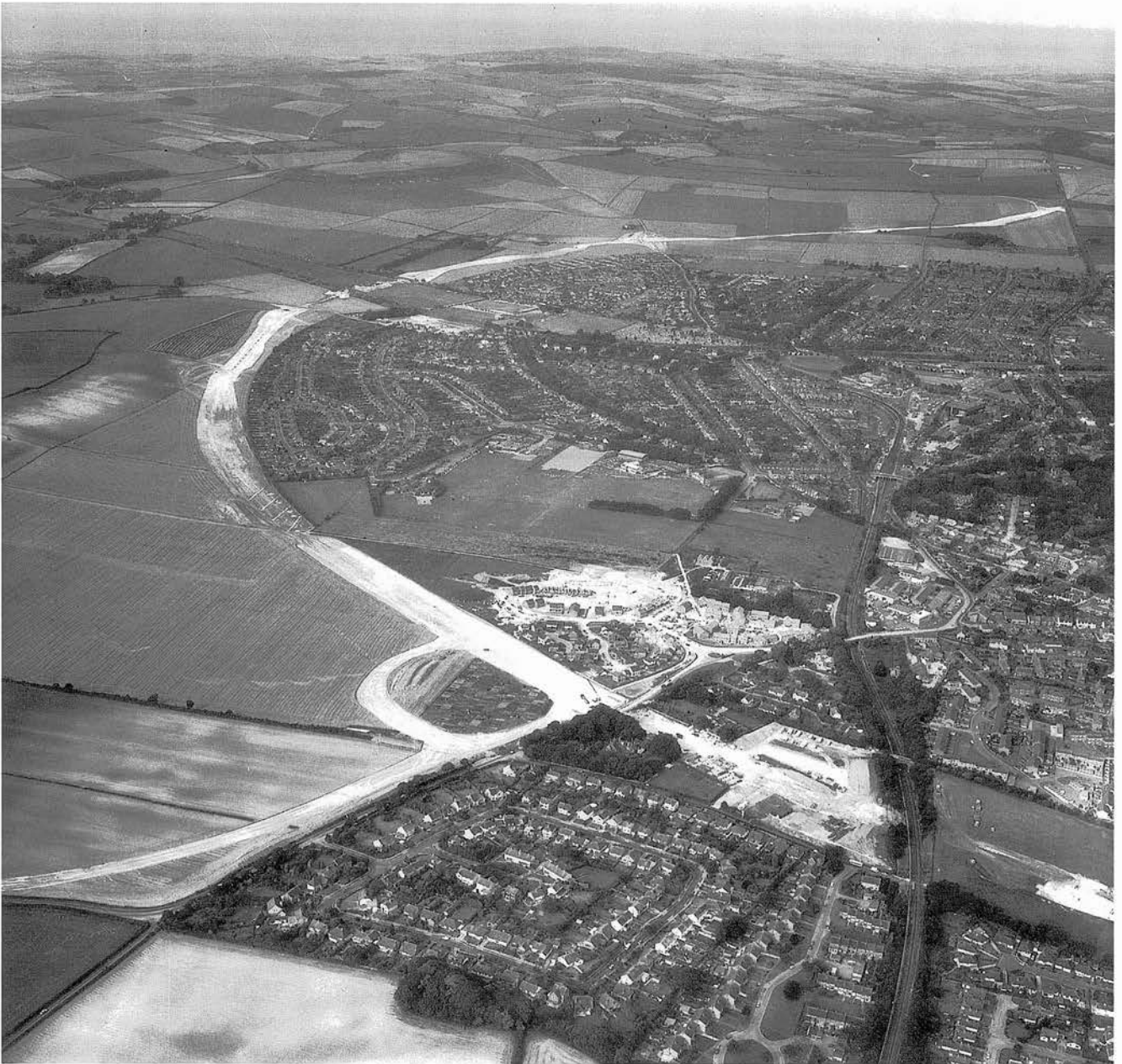
Frontispiece The Dorchester By-pass under construction in late summer 1987. The view is from east to west, with St Georges Road (Site 2) and Flagstones (Site 3) in the bottom right, around to the Bridport Road Ridge (Site 9) in the top right. Conquer Barrow is hidden in the clump of trees at bottom centre. Maiden Castle and Maumbury Rings are clearly visible. (RCHM(E) NMR 4002/06, © Crown copyright reserved)
