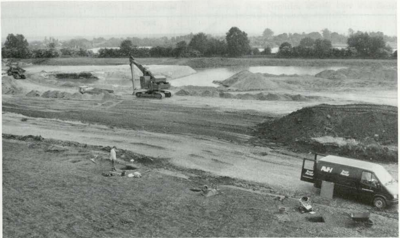
Plate 2 Bray: gravel extraction in progress at the southern end of the site
