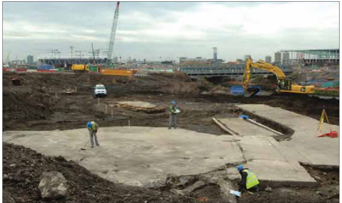
Plate 6.29: World War II Defences showing gun emplacement, Building 4, nissen huts, Buildings 15 and 16 and part demolished service road looking south (BHA 19)
