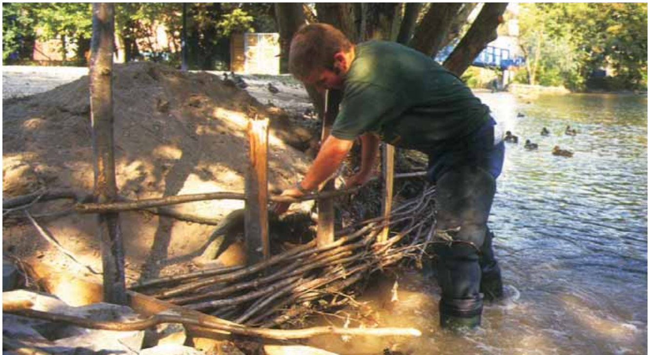
Figure 29: Recent stabilisation of riverbank at Wilton (Wiltshire) using wattle – similar to that found between revetments 1 and 4.
