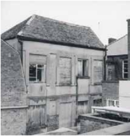
Figure 73: Surviving mid-17th century roof structure to the rear of the northern part of the Castle Inn.
