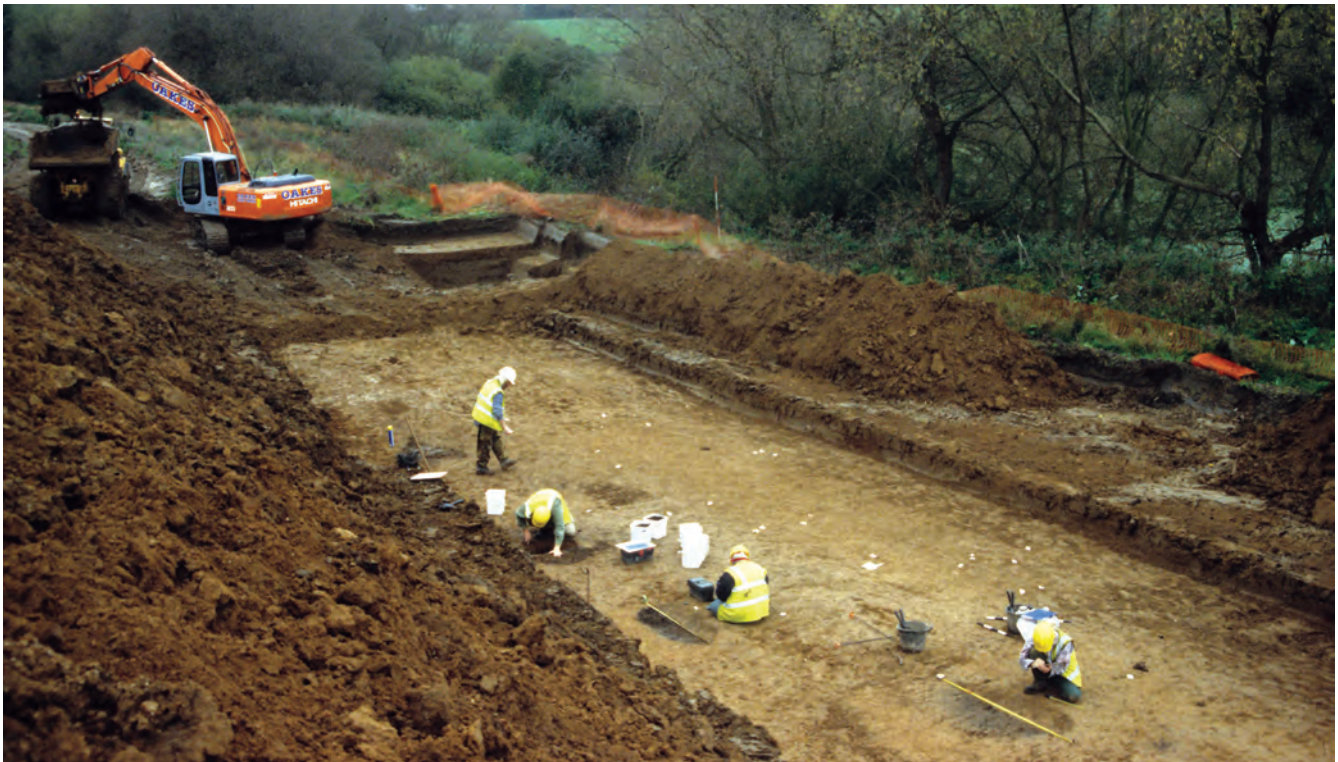
Plate 21.8 Excavation of Early Bronze Age pits at the Ebbsfleet River Crossing (ARC ERC01)
