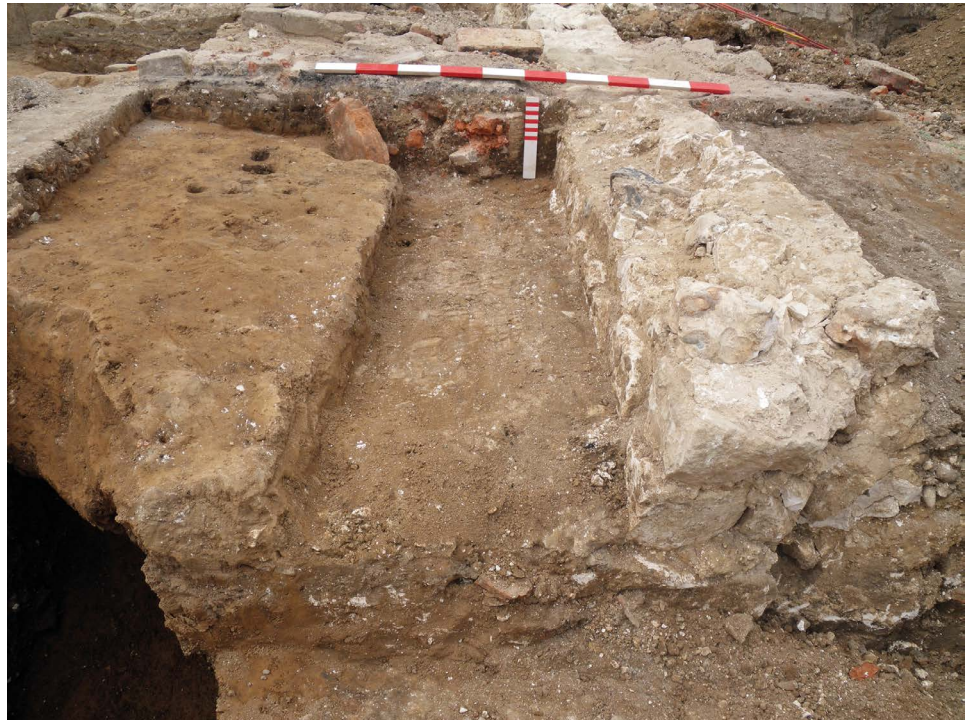
Plate 4.9 Wall foundations of typical domestic dwellings in medieval Salisbury, as seen in Vanner's Chequer (Harding 2016). Scales: 1 m and 0.2 m
