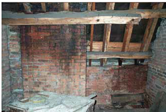
Fig. 35 External pointing in the south wall of the north-west attic room
