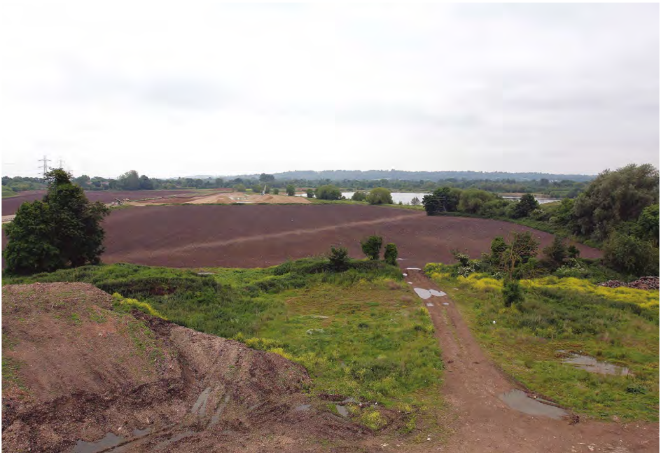
Figure 1.5 Looking south from the Plant Site across the Thames Valley. Excavation along the Conveyor area can be seen underway to the left
